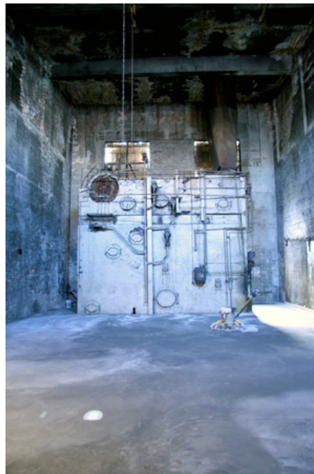
Interior shot of Pierogi's Boiler.
